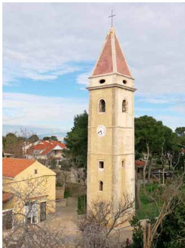
2. Pogled na zvonik s jugozapada (foto: E. Motušić) View of the bell tower from the south-west
